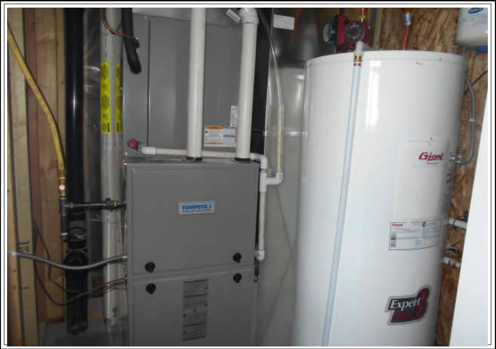
Basement - mechanical room
